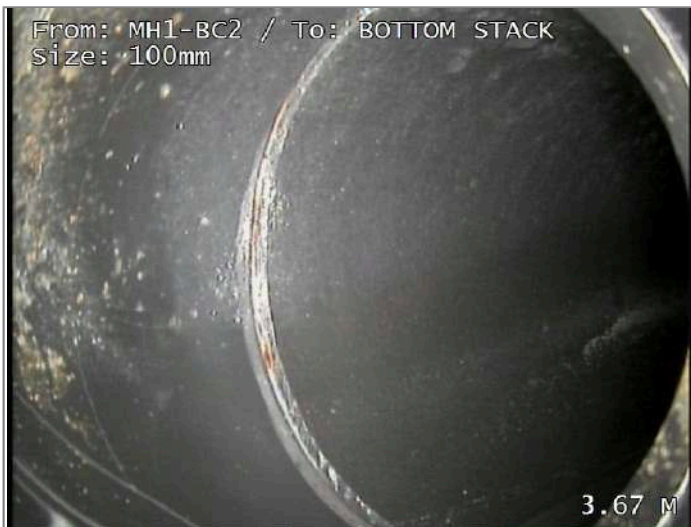
Line of drain/sewer deviates right
