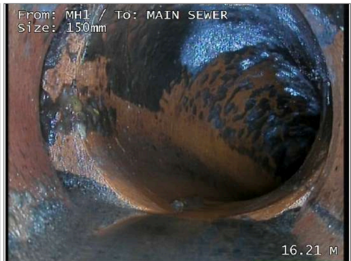
Joint displaced 15mm
