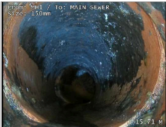
Joint displaced 15mm
